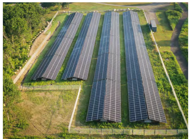
Ground mounted East West ballasted system
