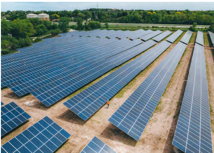
An efficient ground-mounted solar system will be installed close to a building's electrical equipment
