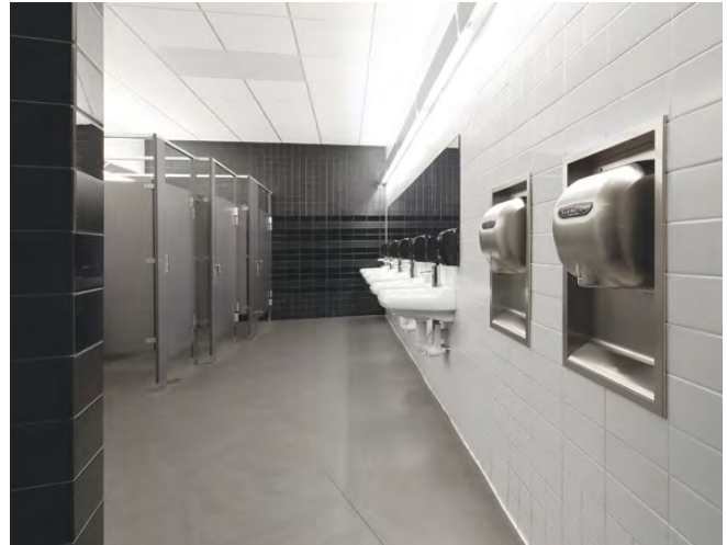
Figure 2. This commercial restroom conveys cleanliness and safety with a row of touchless sink faucets and high-speed, energy-efficient hand dryers
