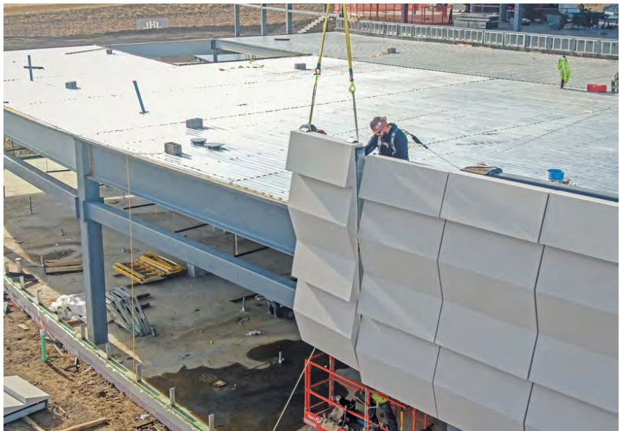
Substantially less structural steel is needed to support the glass fiber reinforced panels compared with what would have been necessary for precast. (IMAGE COURTESY JHL CONSTRUCTORS)
