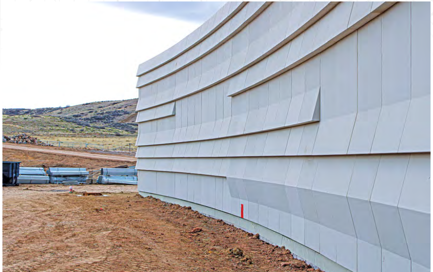
The panels resemble flowing water, and the details in relief interplay with varying levels and angles of sunlight. (IMAGE COURTESY JHL CONSTRUCTORS)
